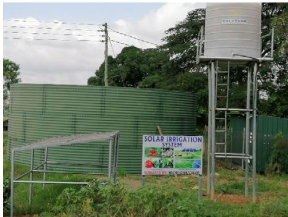
Figure 4: Solar irrigation system at Kwadaso
