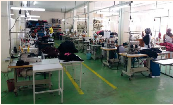
Ferehiwot Garment: the electric cabling has been improved. It used to be on the floor, but the work space is now safer because electricity cables are now leading towards the ceiling.
