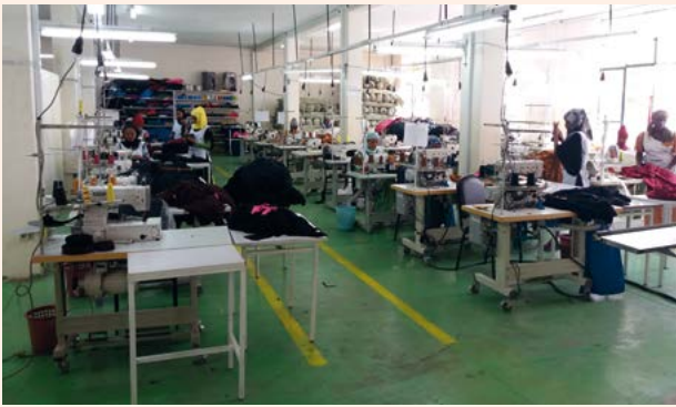
Ferehiwot Garment: the electric cabling has been improved. It used to be on the floor, but the work space is now safer because electricity cables are now leading towards the ceiling.
